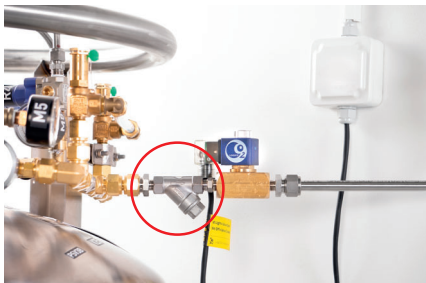
Enrichment Valve installed with filter
